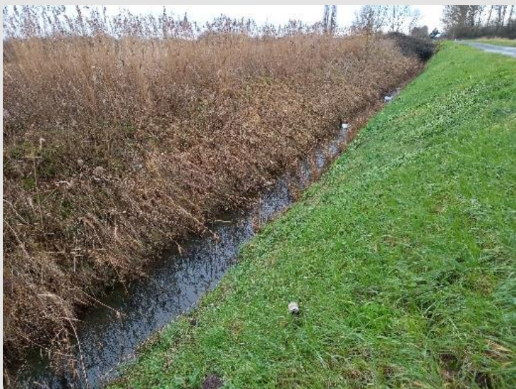
TF 45425 07733 View of IDB adopted drain, which flows along the southern edge of New Bridge Lane (between nodes 43 and 44). Image captured from the culvert, which provides vehicular access to the field to the south, facing West.
